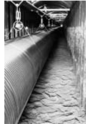
The laser beam runs through an evacuated tube in order to avoid perturbations from air pressure fluctuations. The vacuum tubes of 60 cm diameter and 0.9 mm wall thickness are suspended in a trench.
